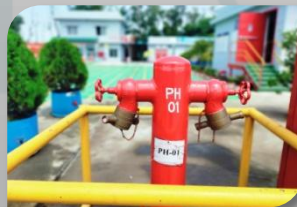
FIRE HYDRANT LINE With 54500 USG Water reservoir
