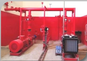
FIRE PUMP (Electrical, Diesel & Joky) 750 GPM Fire Pump Set Approved by FSCD
